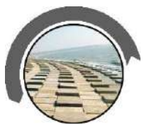
Erosion Conc. Blocks
