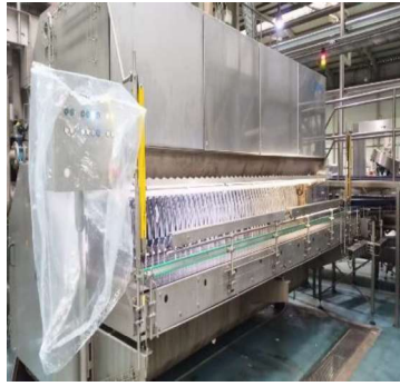
Figure 72 - Maintenance at the outlet of the bottle washer.
